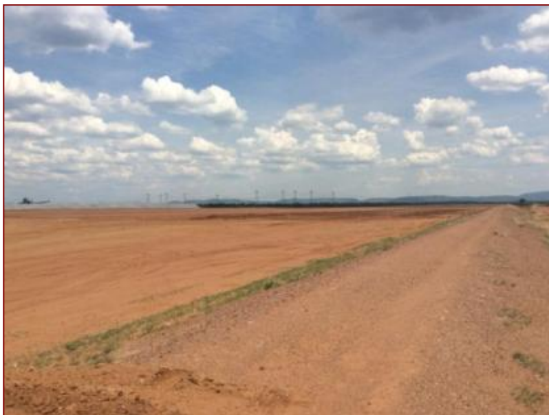
Figure 17- Available land that has been cleared for the growth of the Ash Disposal Facility (AFD). Image taken from the west facing east
